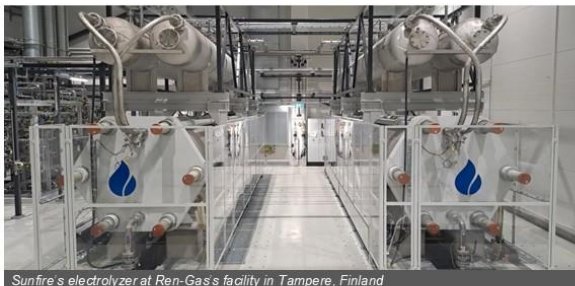
Sunfire's electrolyzer at Ren-Gas's facility in Tampere, Finland
