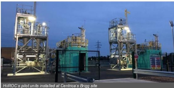
HiiROC's pilot units installed at Centrica's Brigg site
