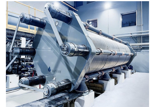
Sunfire 10MW alkaline electrolyser stack
