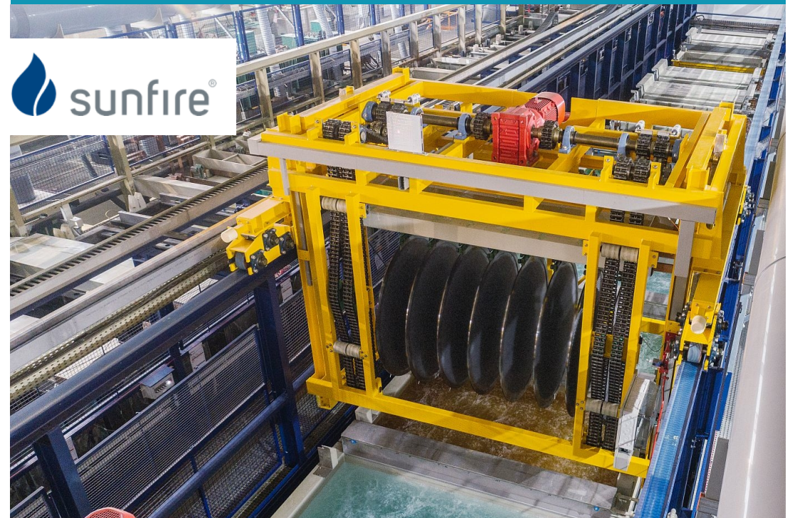
Sunfire's alkaline electrolyser plant in Solingen, Germany
